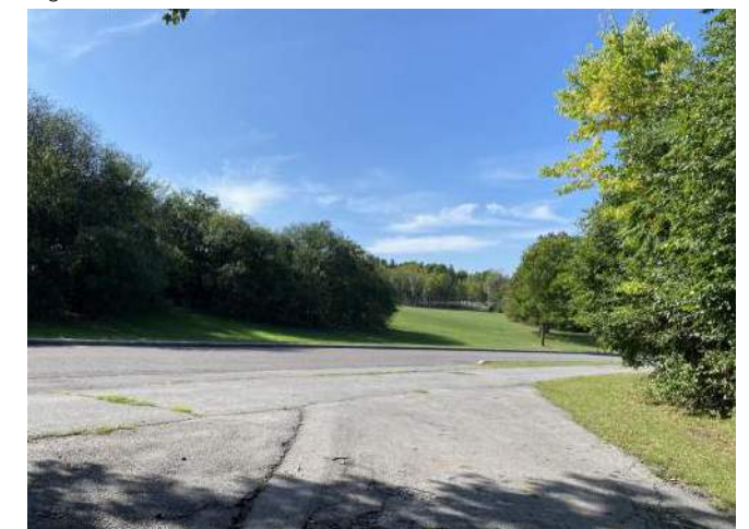
The margins of roadway and pedestrian/bike path, show multiple layers and excessive pavement
