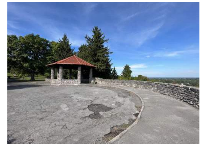
Pavement near the Pinnacle is showing signs of wear and cracking. Pedestrianization of this zone should be considered
