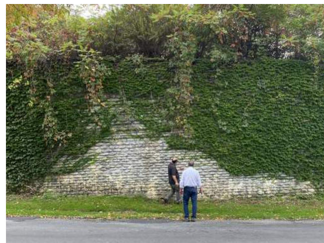
Existing retaining wall exhibits calcium efflorescence
