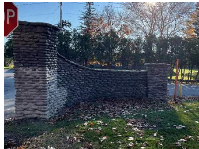
Grout not consistently colored on masonry walls
