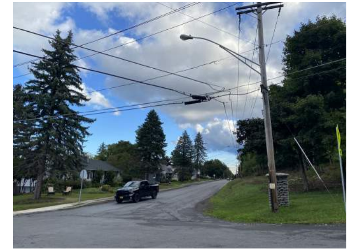
+ Street Lights - Wooden Pole
