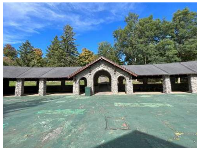
Interior pavement and event access to the Former Horse Pavilion/ Picnic Pavilion need improvement.
