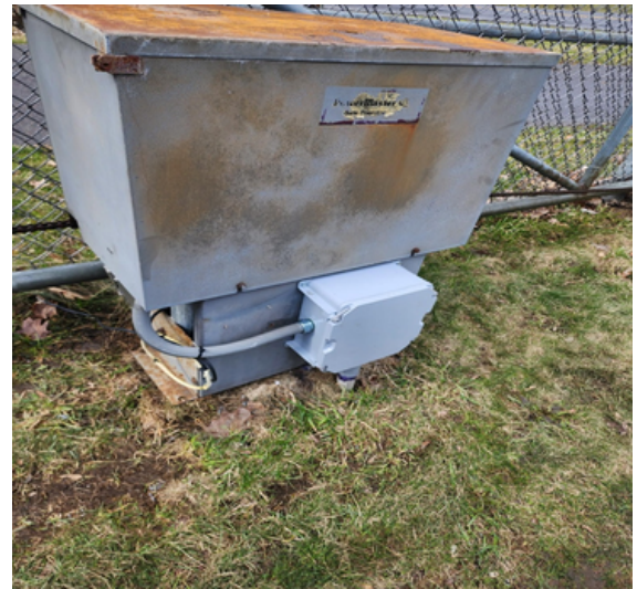
New watertight electrical enclosure installed
