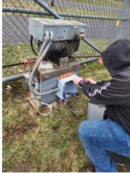
Electrical control box damage identified
